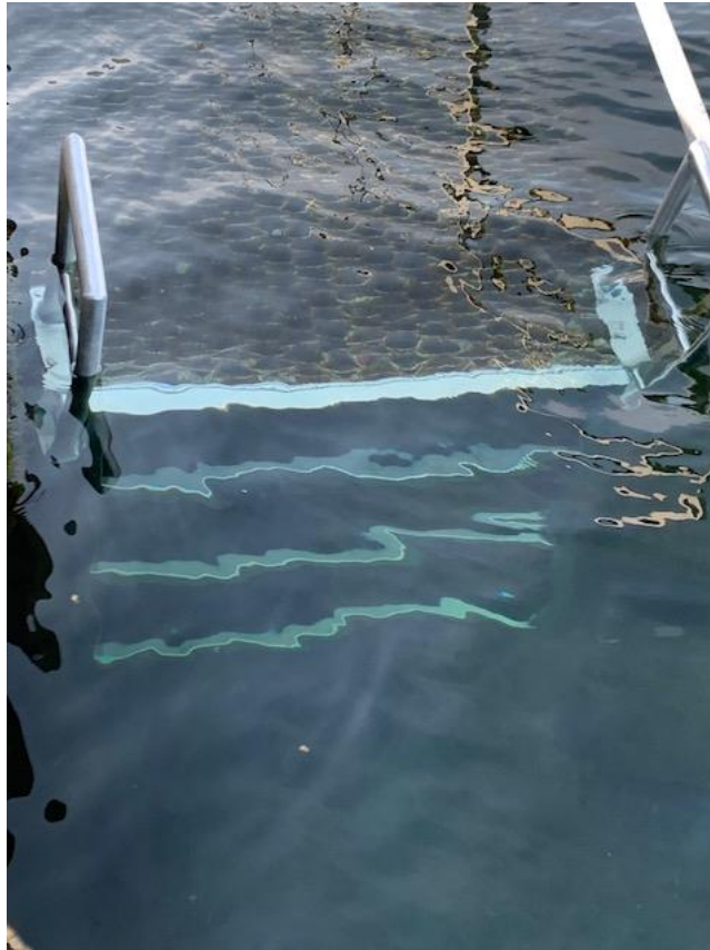
New swim ladder installed on the ramp at the Prescott Scuba Park.
